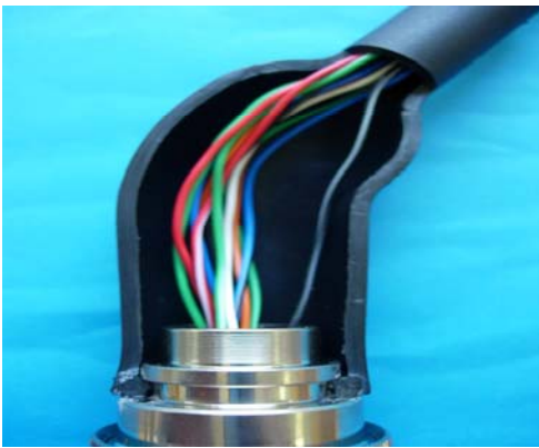
NOT ACCEPTABLE Insufficient strain relief on all wires
